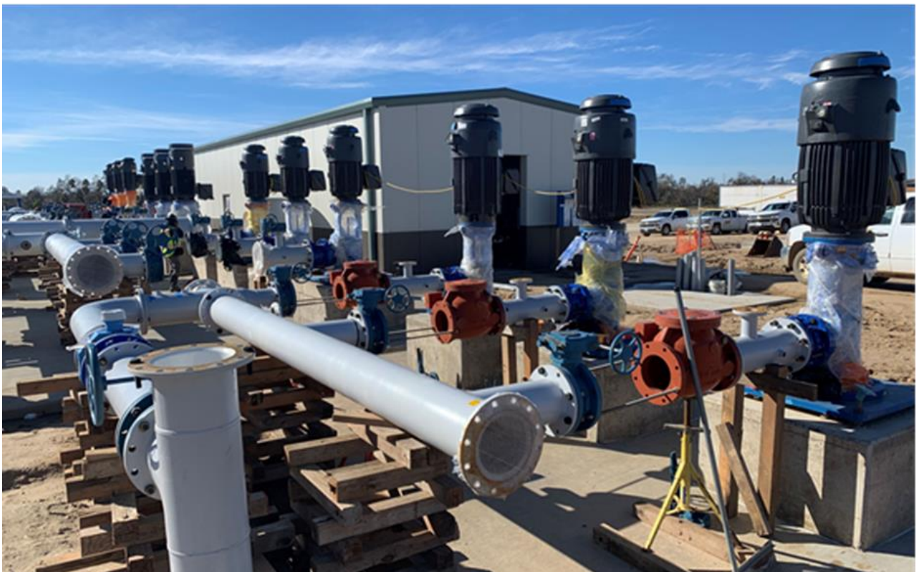
Finished Water Pumps
