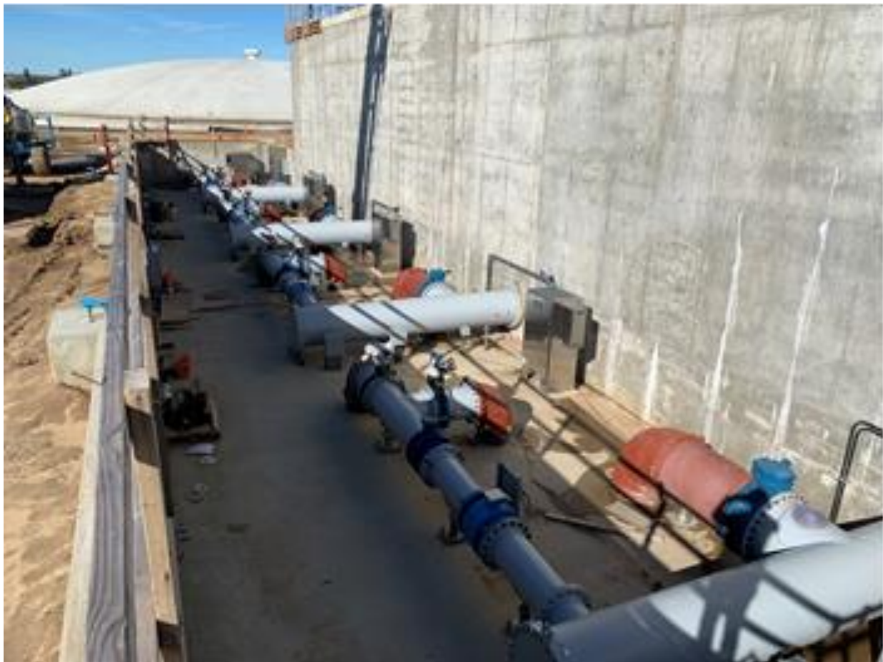
Ozone and Filter Piping
