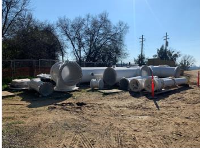
Raw Water Pump Piping
